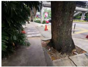
Inconsistent width of walkway. Presence of physical obstruction (tree)
