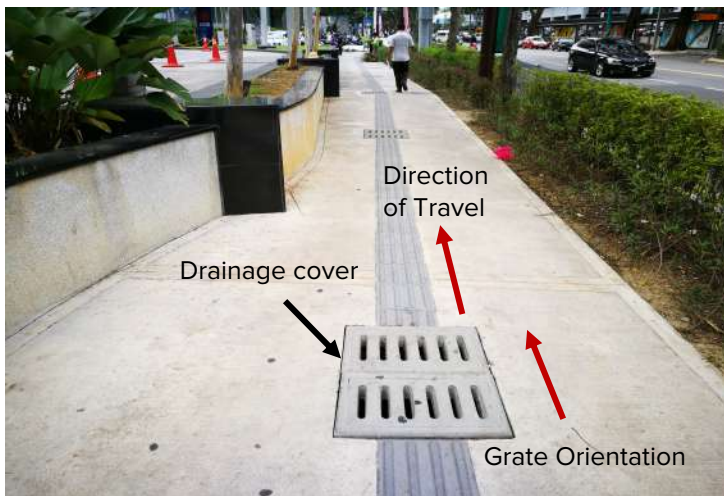
Photo 4.4: Example of incorrect placement of drainage/stormwater cover
