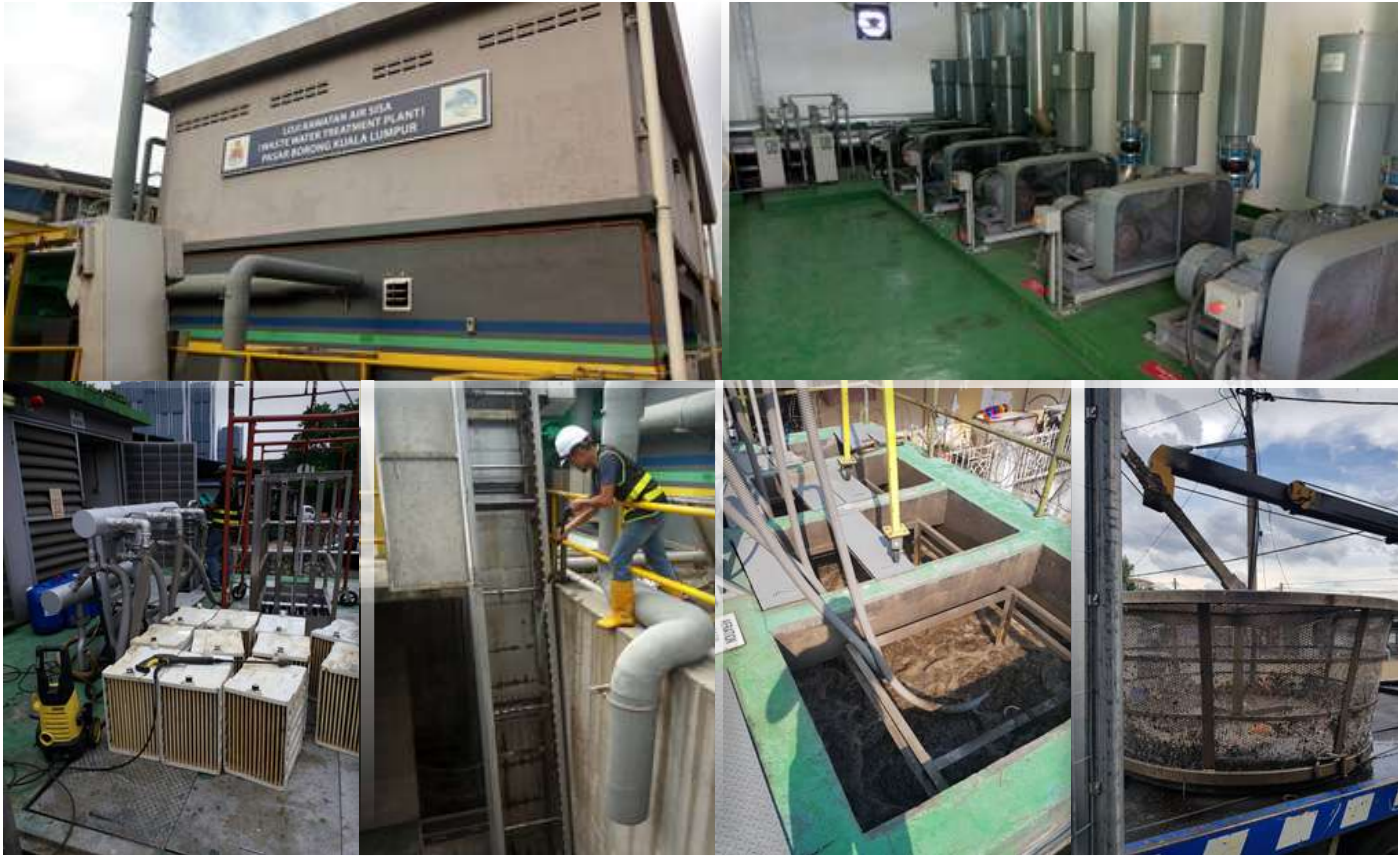
Waste Water Treatment Plant
